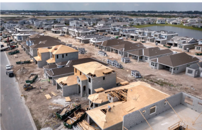
Homes being built on the second phase of the Minto Orchards community on February 25, 2023. GREG LOVETT / THE PALM BEACH POST
